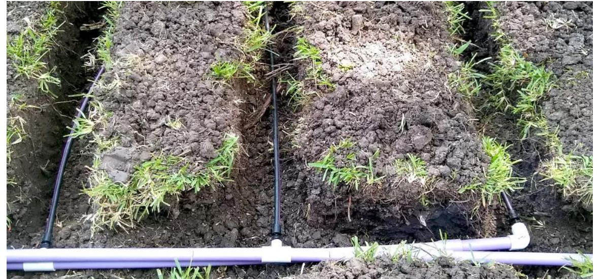
Figure 2: Example of a drip irrigation septic water disposal system, Parker's Septic Services
